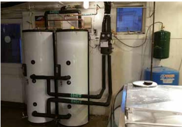
Hamley Farms | Barton, NY | Storage Tanks
